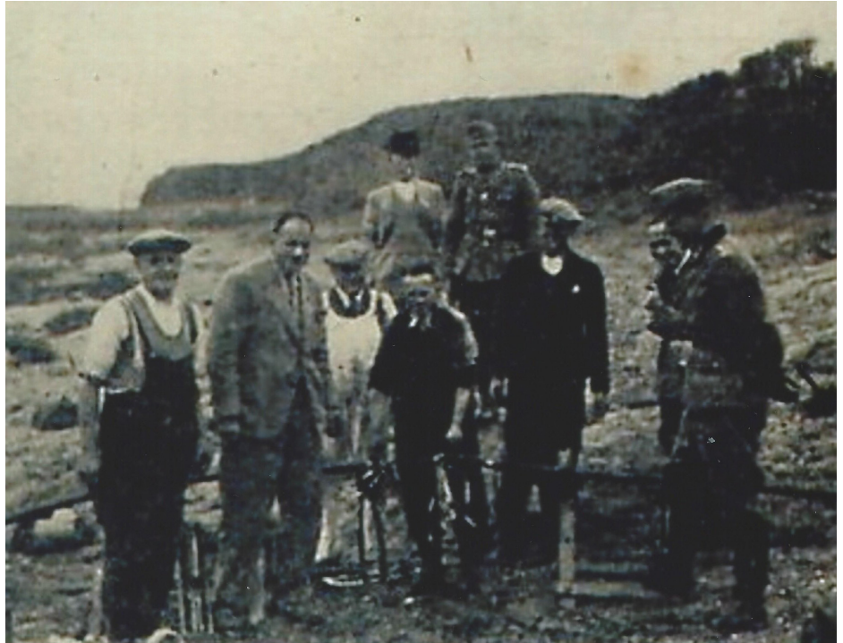
■ Phil and members of the Telephone Department jointing team, under German supervision, reconnecting the submarine cable at Fliquet Bay
